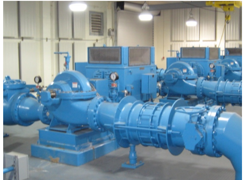
Hesperian Pump Station
