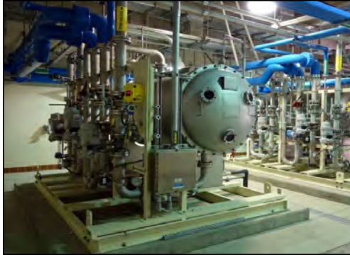
Upgraded and Increased Dosage for 120 MGD of Ozone and Peroxide Capacity (USL and Sobrante WTPs)
