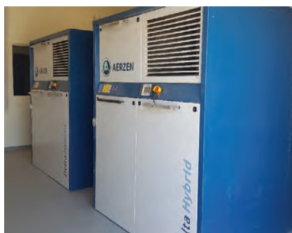
Two hybrid rotary-lobe blowers (Aerzen USA) serve each oxidation ditch, providing redundancy.
