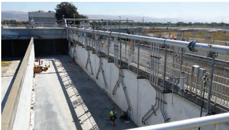
New fine-bubble aeration with automated dissolved oxygen control helps drive down energy costs significantly.
