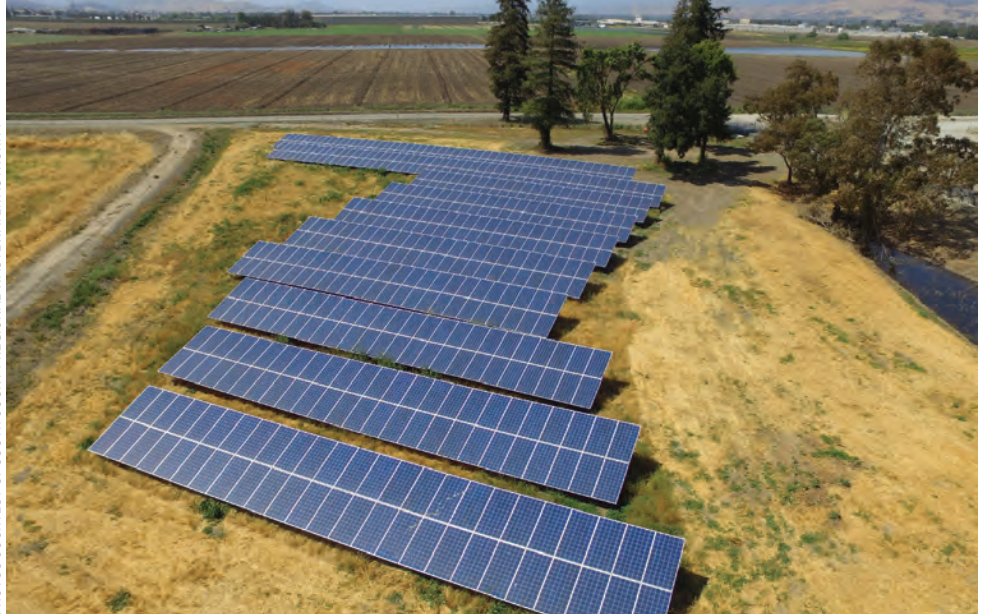
This 190 kW solar array powers the influent pump station at the South County Regional Wastewater Authority treatment plant and exports surplus power to the utility grid.
