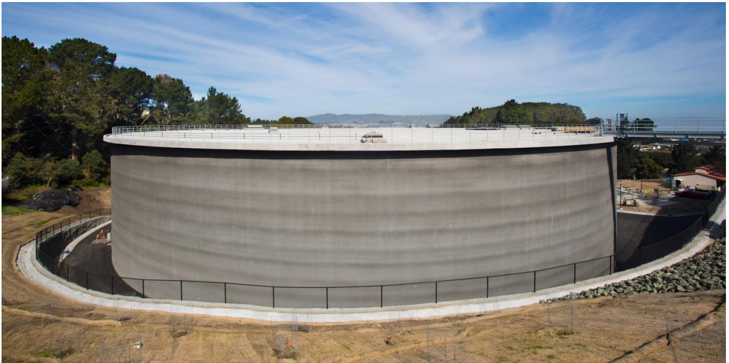
Treated water reservoir
