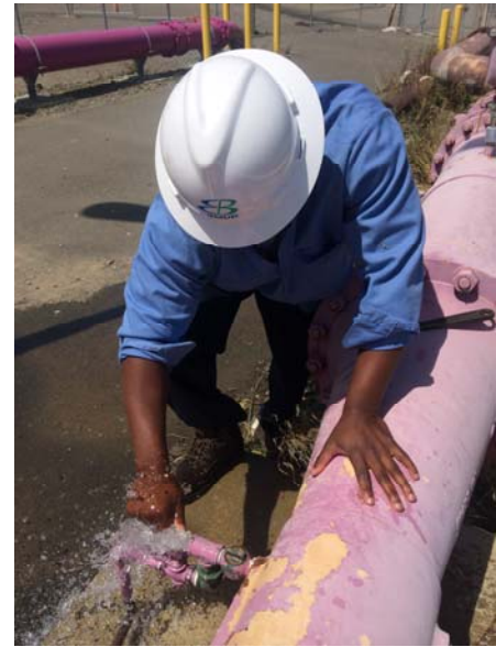
Figure 5.4: East Bay Municipal Utility District intern performing preventative maintenance on the recycled water system.
