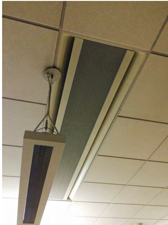
Chilled Beam in a classroom in LA/SS building. Photo Credit: Krishnaveni Meka
